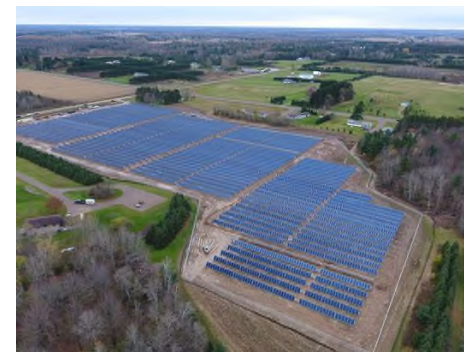
A large solar field built for Dairyland Power Cooperative in Medford. (Photo: Courtesy of Renew Wisconsin)
