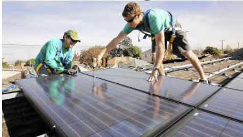
Solarcity workers Joey Ramirez, left, and Taran Stone install solar modules on the roof of a Long Beach home. (Al Seib / Los Angeles Times)
